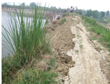
图 2 民乐水库副坝滑坡 Fig.2 Auxiliary dam landslide of the Minle Reservoir
