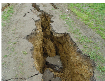
图 1 新油房水库大坝裂缝 Fig.1 Dam crack of the Xinyoufang Reservoir
